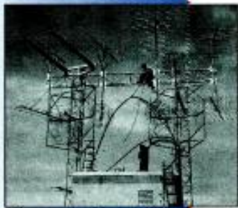
Microwave antenna tower
